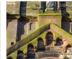
Greater material staining
