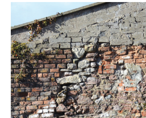
Accelerated material degradation
