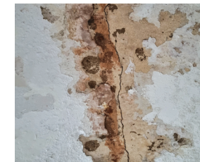
Increased water ingress and damp
