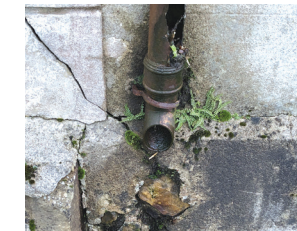
Higher likelihood of rainwater goods failure
