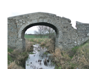
Deterioration of existing infrastructure
